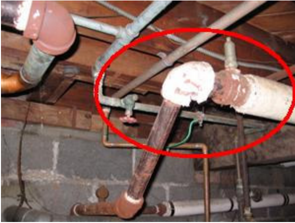
13.5 Picture 1 Heating pipes
