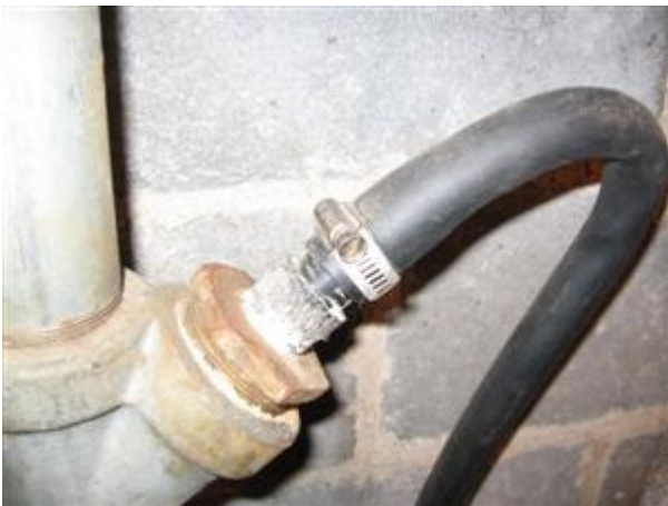
8.7 Picture 1 Washer drain
